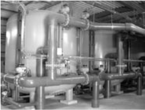
Figure 6.2. Steel tower sand filters (Photograph from I. Smit)
