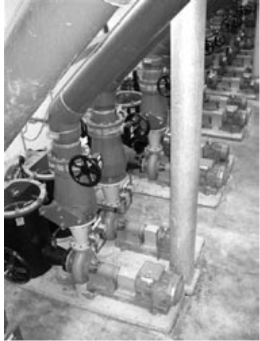
Figure 6.1. Pumps and pre-filter baskets (Photograph from I. Smit)
