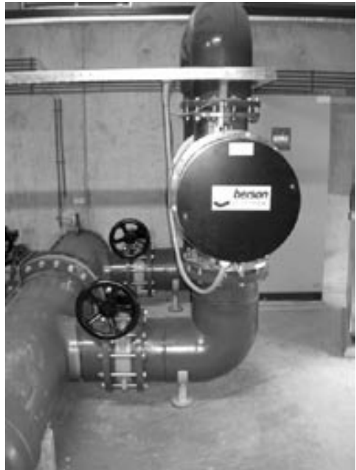
Figure 6.8. UV unit (Photograph from I. Smit)
