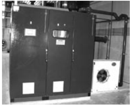
Figure 6.6. Ozone control cabinet (Photograph from I. Smit)
