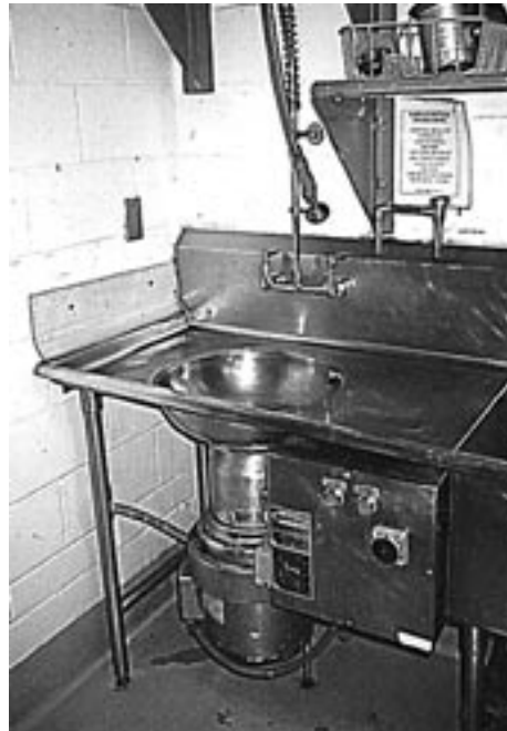
Figure 7.2. Grinder under sink
