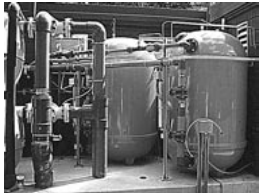
Figure 6.7. Small ozone contact chamber
